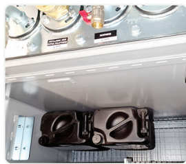
Pump room with extra space for storage of tools and containers
